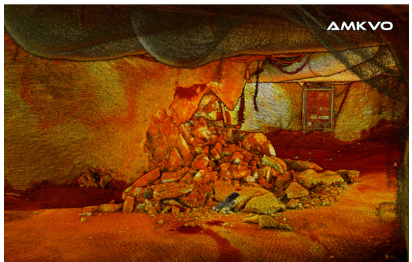
Hovermap is ideally suited to the exploration and mapping of areas affected by a fall-of-ground. In 2019, when LKAB's Kiruna Mine experienced a seismic event, Emesent partner AMKVO mapped kilometers of damaged drifts in just a few days.
